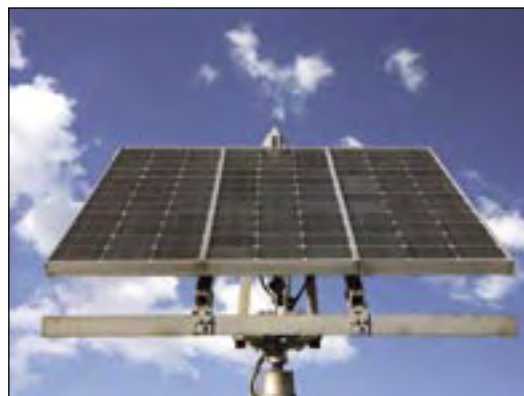
Solar Photovoltaic (PV) System
